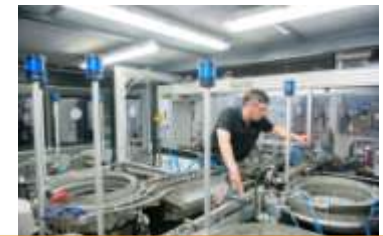
Maintenance and Service
